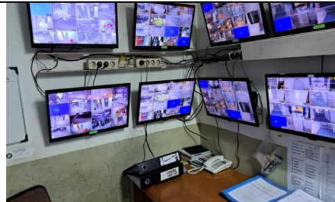
Monitor CCTV Swissbel Residence Rasuna Epicentrum
